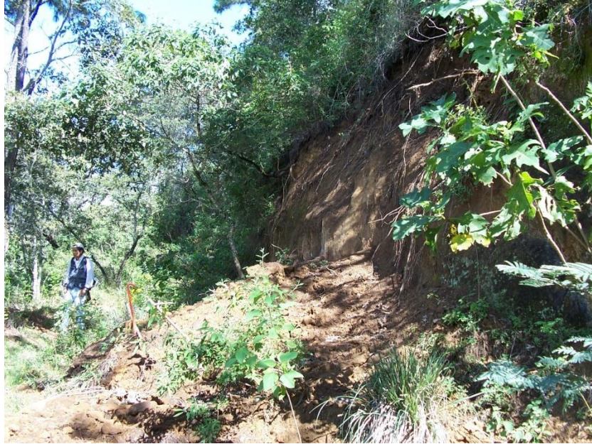
Figure. 1. Example of detachment in a vertical section of a sidewalk at the top of Parque las Peñas
